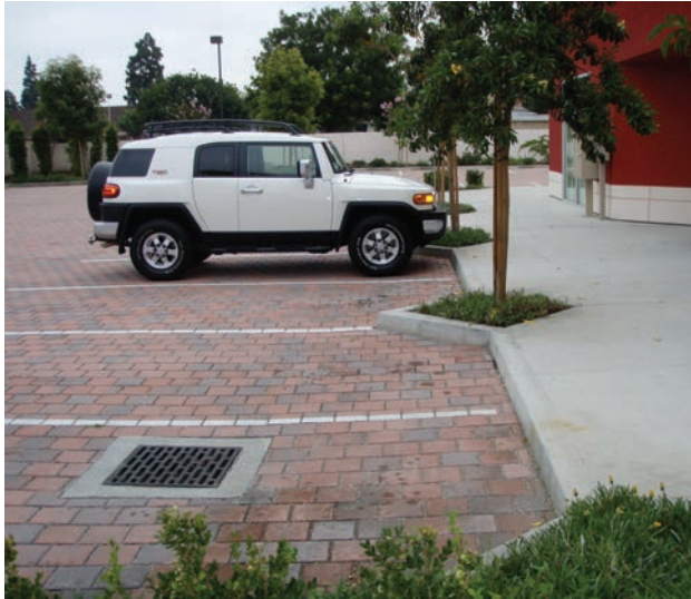
Pervious paving with pea gravel over an infiltration area.
