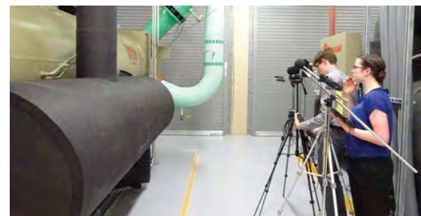
Figure 10. Acoustical measurements and recordings of the chillers and pumps inside an existing facility similar to the proposed central energy plant.
