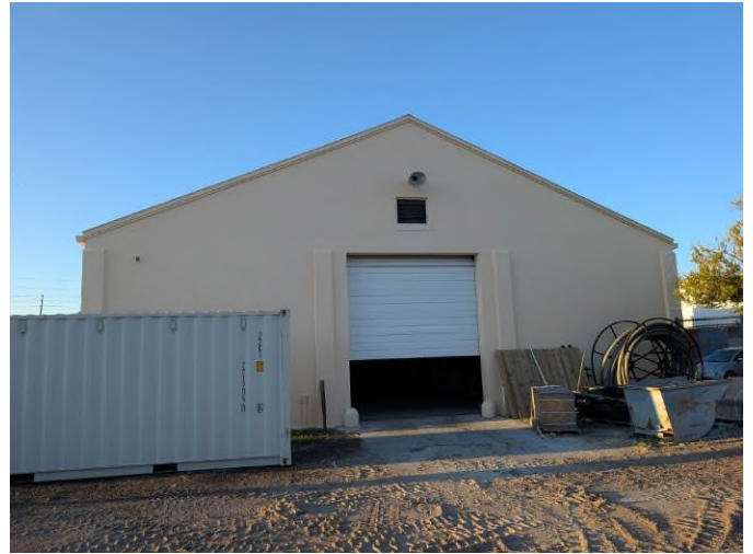
View of A/C Units
