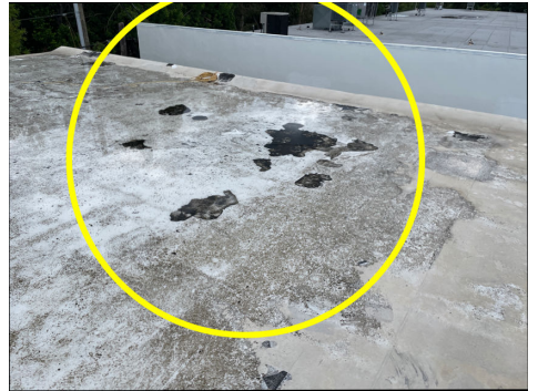
Damaged/Loose roofing material(s) were visible at multiple locations. An evaluation and repair should be completed by a qualified licensed roofer.
