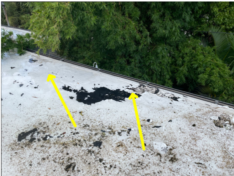
Damaged/Loose roofing material(s) were visible at multiple locations. An evaluation and repair should be completed by a qualified licensed roofer.
