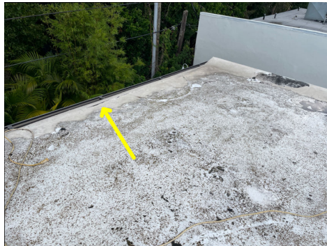
Damaged/Loose roofing material(s) were visible at multiple locations. An evaluation and repair should be completed by a qualified licensed roofer.
