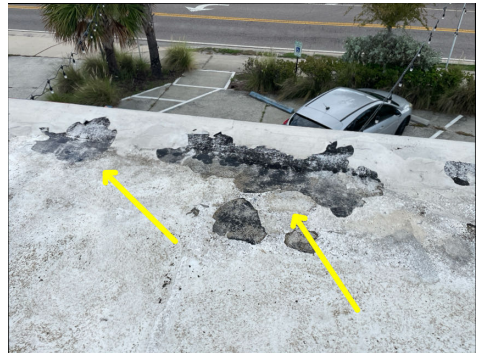
Damaged/Loose roofing material(s) were visible at multiple locations. An evaluation and repair should be completed by a qualified licensed roofer.
