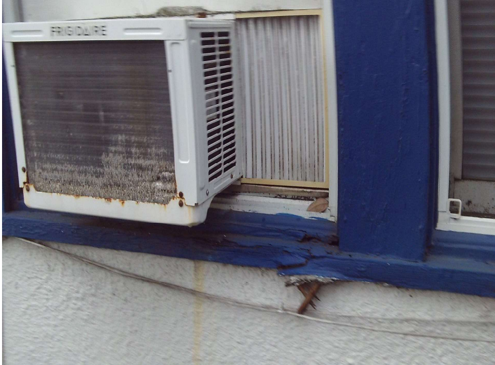
MINOR WOOD DAMAGE, OFFICE EXTERIOR WINDOW
