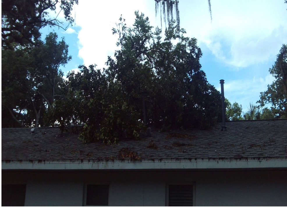
TREE LIMBS OBSERVED ON ROOF OF BUILDING 100
